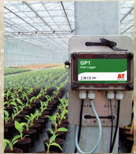
GP1 Data Logger controlling precision gantry irrigation within a glasshouse at Hillier Nurseries.
